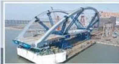
The Cross Bay Link bridging Lohas Park in Tseung Kwan O with Lam Tin has an infinity arc central span that must have been heavy for the floating cranes.
