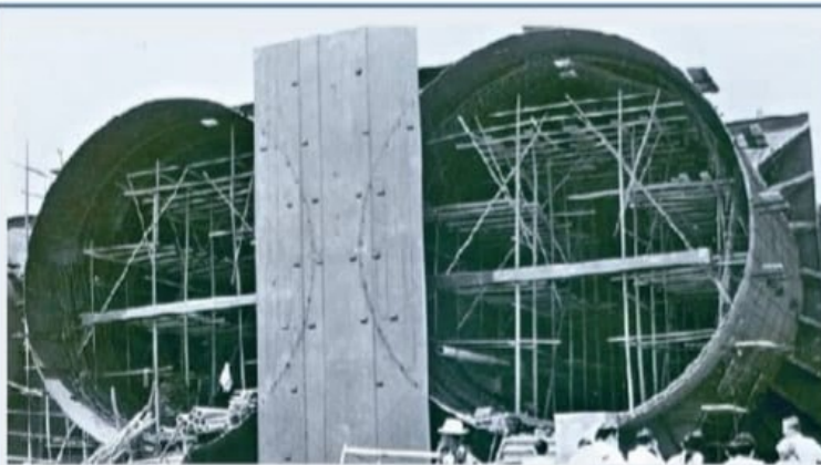
The Cross-Harbour Tunnel, opened in 1972, was designed in round steel sections. SING TAO
